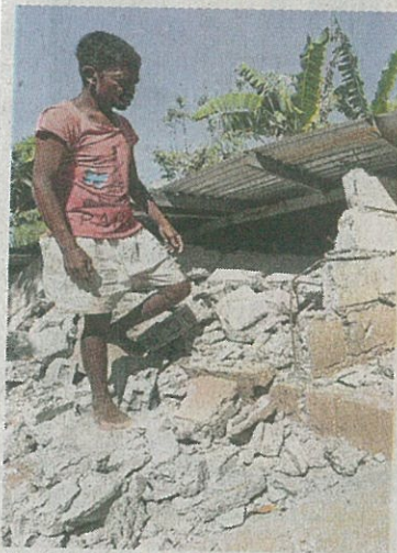
QUAKE DAMAGE An Aeta resident in Floridablanca, Pampanga, checks his house after it crumbled when a 6.1-magnitude earthquake struck in April. —GRIG C. MONTEGRANDE
